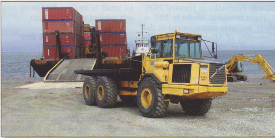
PRL arrives at Cape Lisburne with containers and equipment for packing and transport of PCB-contaminated soil and debris.
